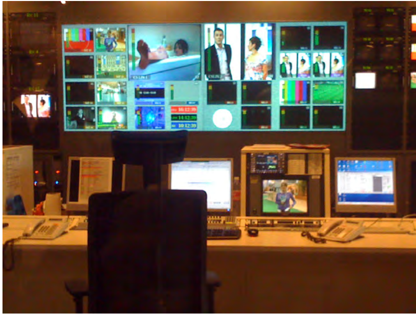
Figure 6: Production-control room at the EiTb TV station
